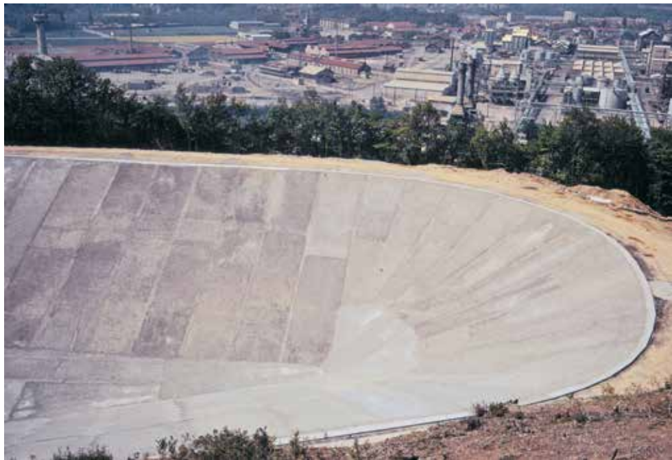
FIGURE 8 Completed leakage collection layer: The chemical plant is on the horizontal ground, 56m below the crest of the reservoir.
