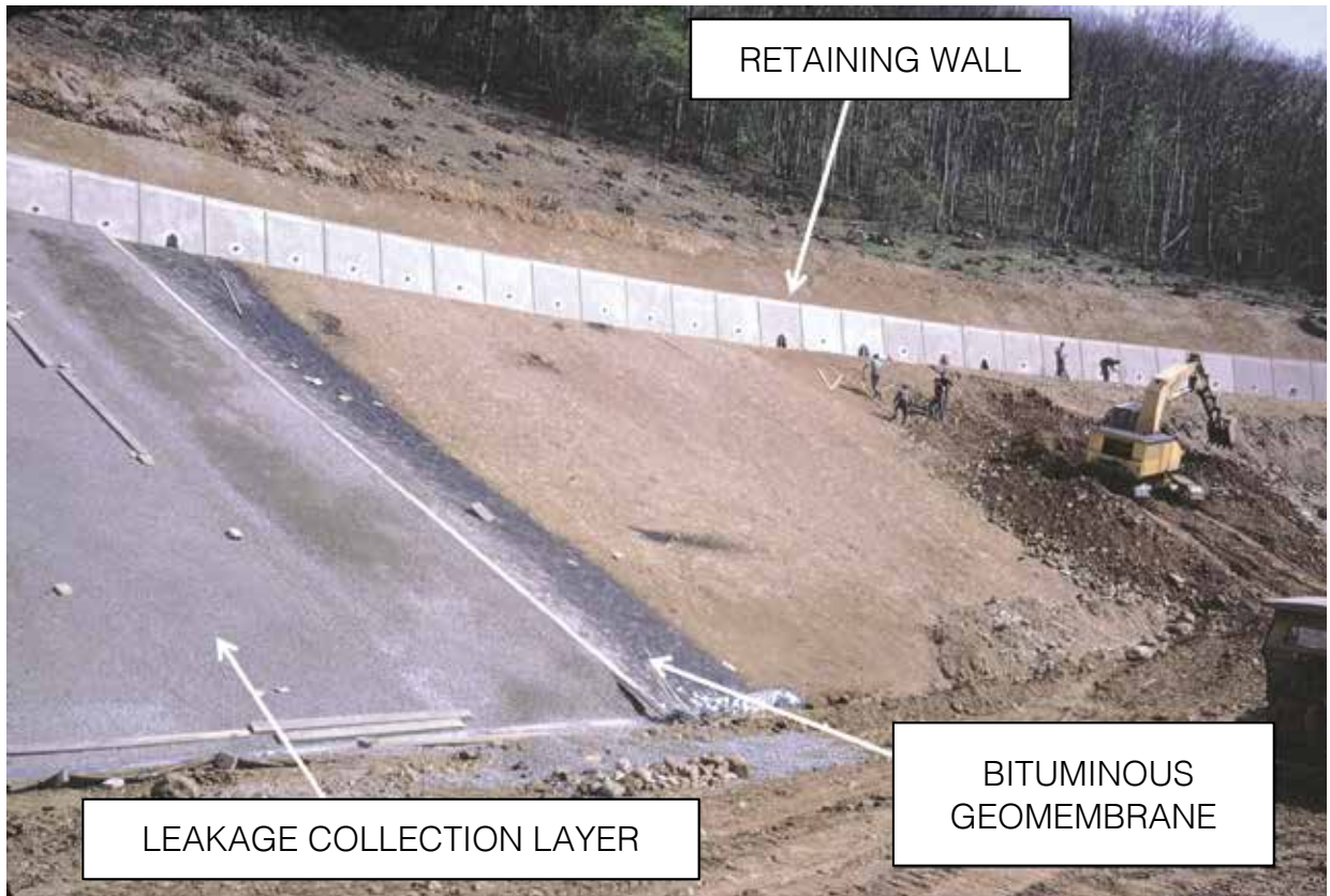
FIGURE 6 Construction in progress with the leakage collection layer directly on top of the bituminous geomembrane.
