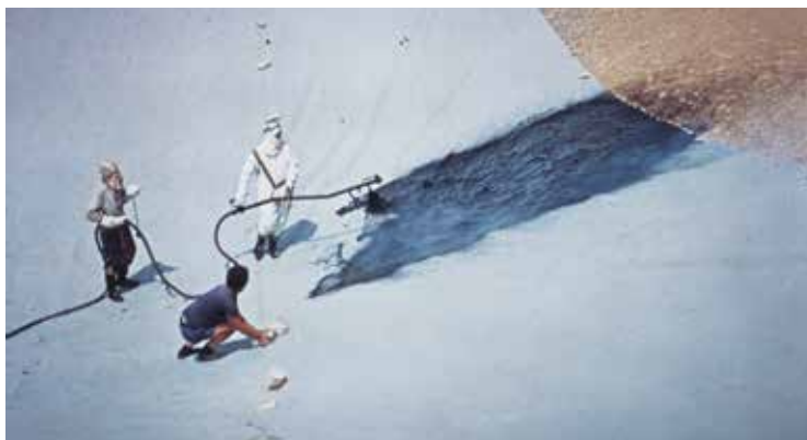
FIGURE 5 Spraying of hot bitumen on a polyester, needle-punched, nonwoven geotextile (photo taken at another site).
