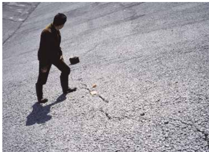
FIGURE 9 Cracks in the leakage collection layer due to some sliding of the gravel layer on the slippery bitumen surface.
